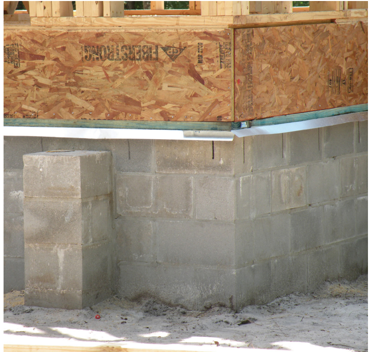
The continuous stem wall foundation, constructed from eight-inch CMU blocks over a poured-in-place footing, encloses the crawl space.
